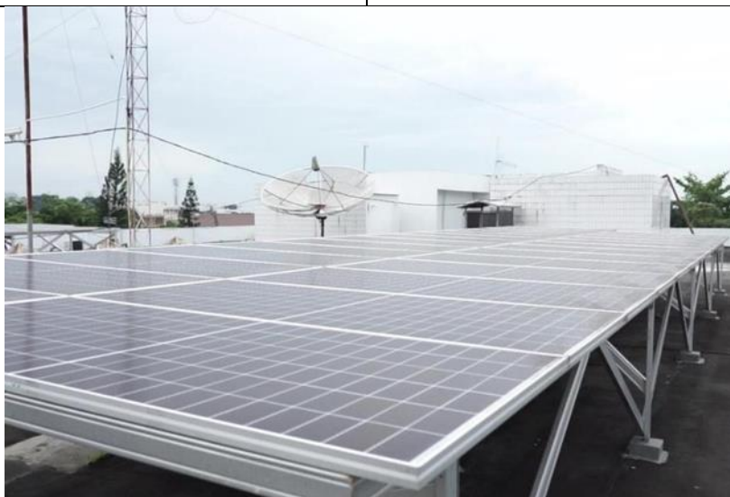
Roof Top Solar Panels in USU Office 21 kWp
